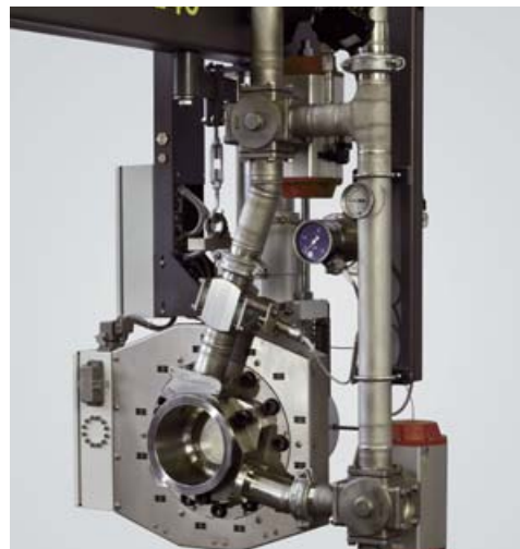
Process water piping
